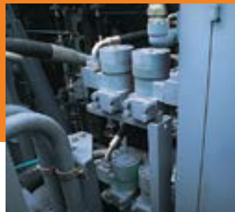
■ The centralized filter system makes inspection and maintenance quicker and more convenient.
